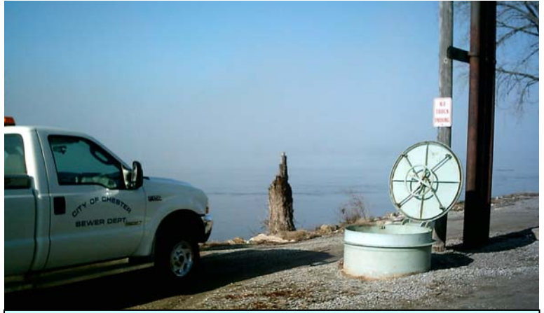
Chester, IL Watertight Lift Station next to the Mississippi River.
