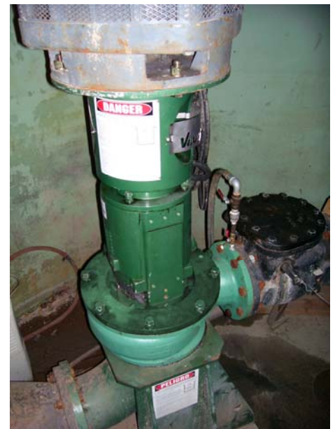
1 of 2 retrofit Vaughan pedestal chopper pumps with older motors.
