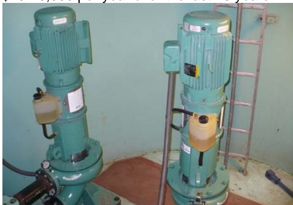
2 of 3 retrofit Vaughan pedestal chopper pumps.
