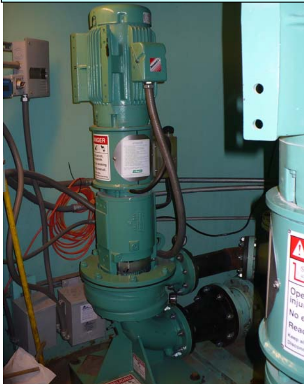
1 of 3 Vaughan Chopper Pumps now installed at the IHCD Taney Lift Station.
