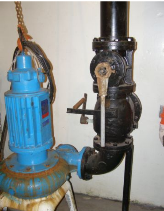
1 of 2 non-clog pumps originally installed
