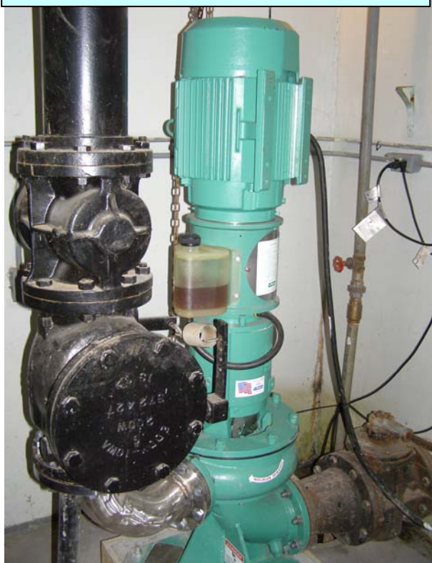
1 of 2 Vaughan Chopper Pumps now installed
