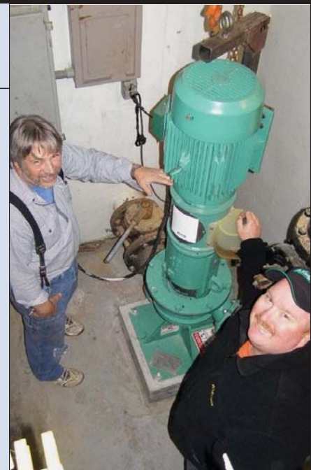
Shown with the chopper pump from Vaughan Company are Greg Fischer, wastewater electrician for the Chehalis Public Works Department (left), and Greg Boone, lead wastewater collection technician.
