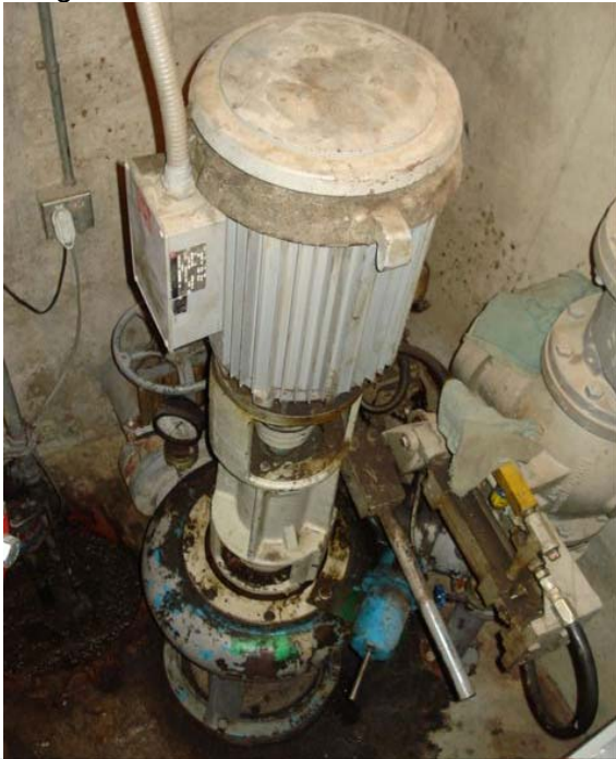
1 of 2 non-clog pumps originally installed
