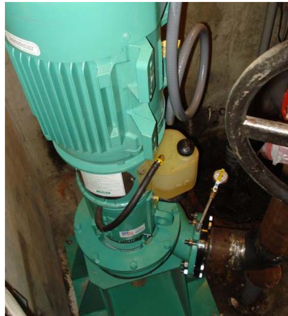
1 of 2 Vaughan Chopper Pumps now installed
