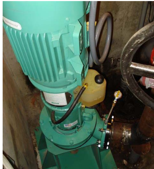
1 of 2 Vaughan Chopper Pumps now installed
