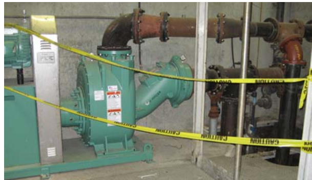
Vaughan 50-HP Self-Priming Chopper Pump drawing about 3500 GPM up 2 pipes from the main influent channel and discharging back into the channel through dual nozzles to create a shearing wall of velocity through which fecal material must flow. Whatever the chopper pump misses, the dual nozzles help to break up.
