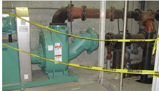
Vaughan 50-HP Self-Priming Chopper Pump drawing about 3500 GPM up 2 pipes from the main influent channel and discharging back into the channel through dual nozzles to create a shearing wall of velocity through which fecal material must flow. Whatever the chopper pump misses, the dual nozzles help to break up.
